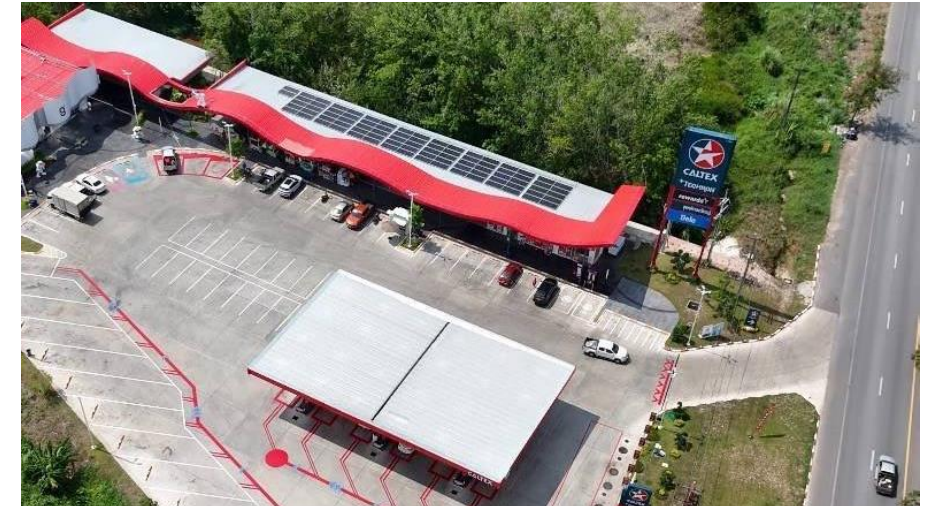
Retail Station Solar Rooftop
