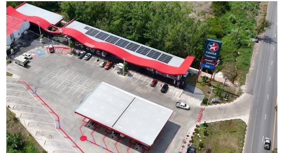
Retail Station Solar Rooftop
